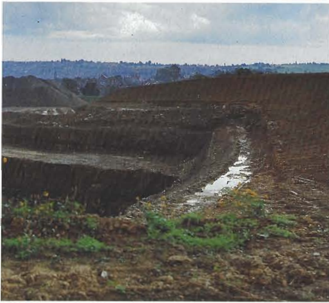
Fig. 29. Mounds of topsoil act as a sight and sound screen around the edge of an active site.
